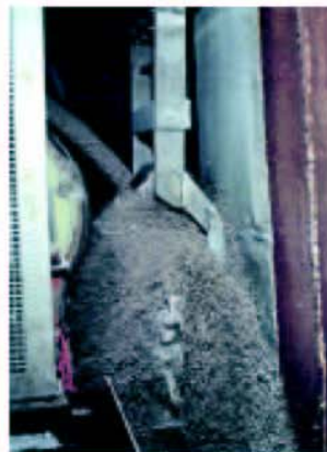
Sampling System for conveyor belt (150 t/h)
